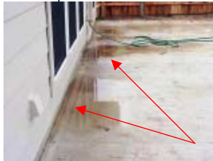
improper drainage at rear patio
