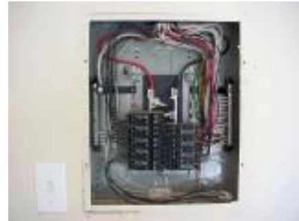
sub-panel in garage
