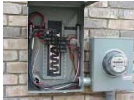
main panel at left exterior
