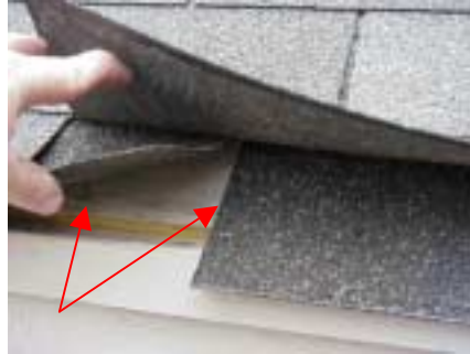
starter course not properly installed felt cut short at drip edge
