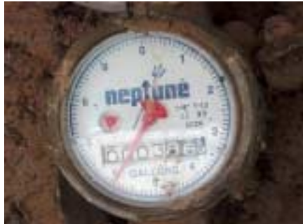
meter indicates that there is a leak in the system
