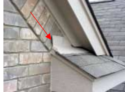
missing counter flashing above front entry
