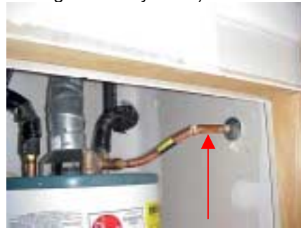
T&P drain line does not gravity drain
