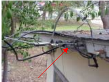
inadequate service attachment
