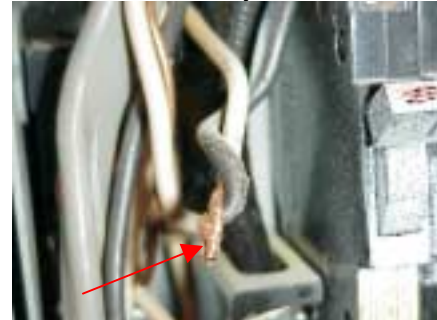
copper wire found with wire nut removed
