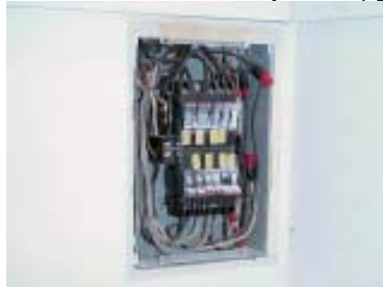
panel box in closet
