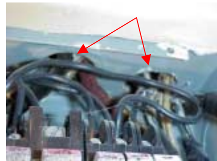
missing bushing protection
