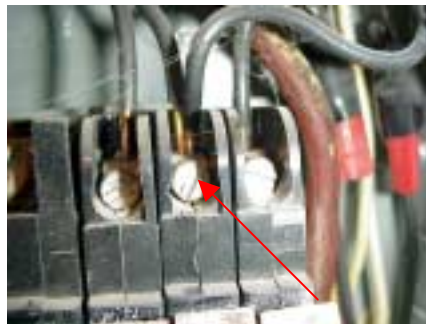
double tapped breaker
