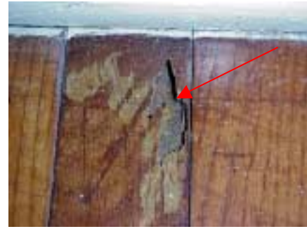
Subterranean Termite damage at floor
