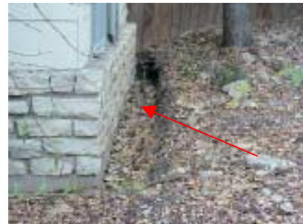
poor drainage at right
