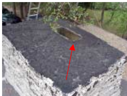
heavy tar coating at chimney / missing spark arrestor and rain cap
