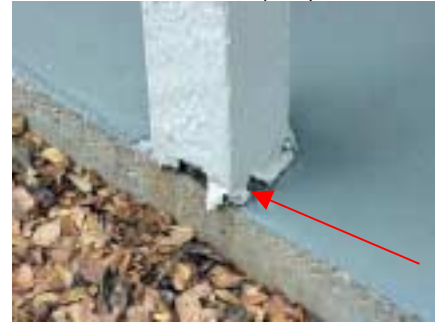
wood rot at carport post
