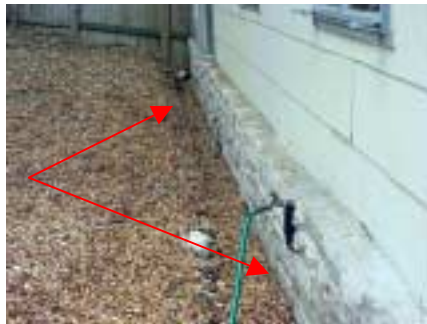
poor drainage at rear
