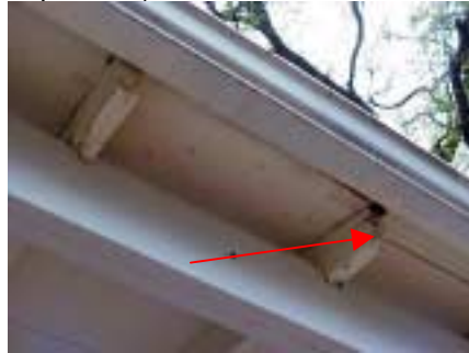
wood rot at carport deck and joists
