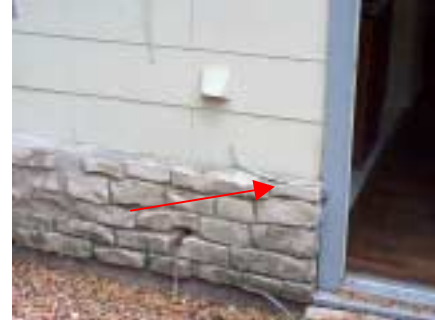
rear exterior wires missing conduit
