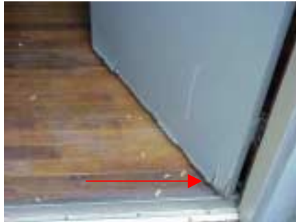
damage are rear exterior door
