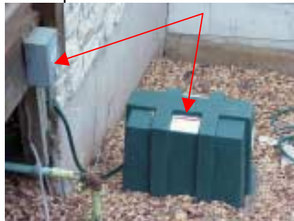
septic system equipment
