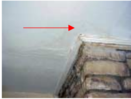
water penetration around chimney
