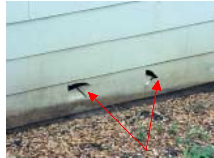
damage at exterior wall tiles
