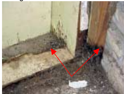
wood rot in wood storage bin
