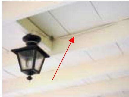
missing conduit at carport light
