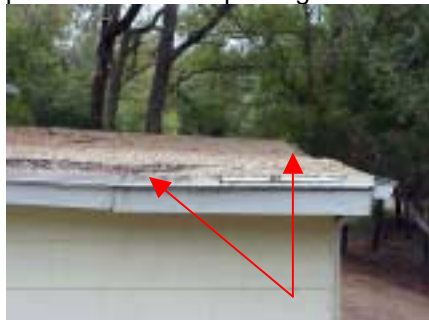
structural issues at carport roof
