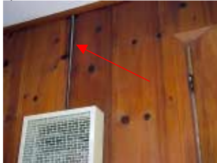
evidence of overheating at panels above furnace
