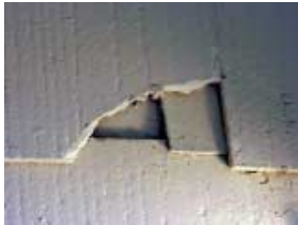
damage at exterior wall tile
