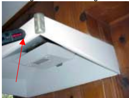
range hood not grounded
