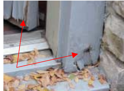
wood rot at rear exterior door / trim
