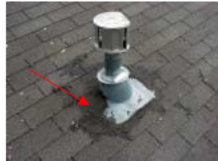
evidence of previous repairs
