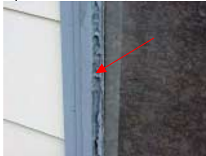
damaged glazing compound
