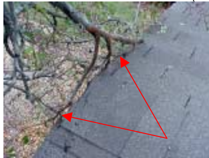
trim limbs / damaged shingles
